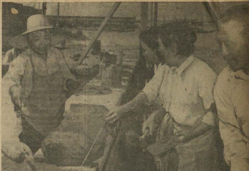
WOMEN BRICKLAYERS —Japanese women help lay the bricks from which adobe buildings are being constructed at the Poston Japanese Relocation Center.
