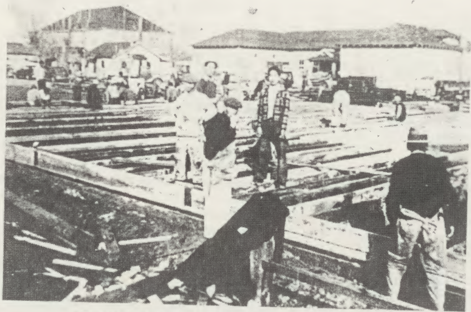
YBA HALL CONSTRUCTION Members of the Buddhist Church working on the foundation of the YBA Hall in January 1939.
