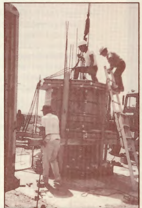
Monument form in place. Ted inspects for true position with Sid Arase.
