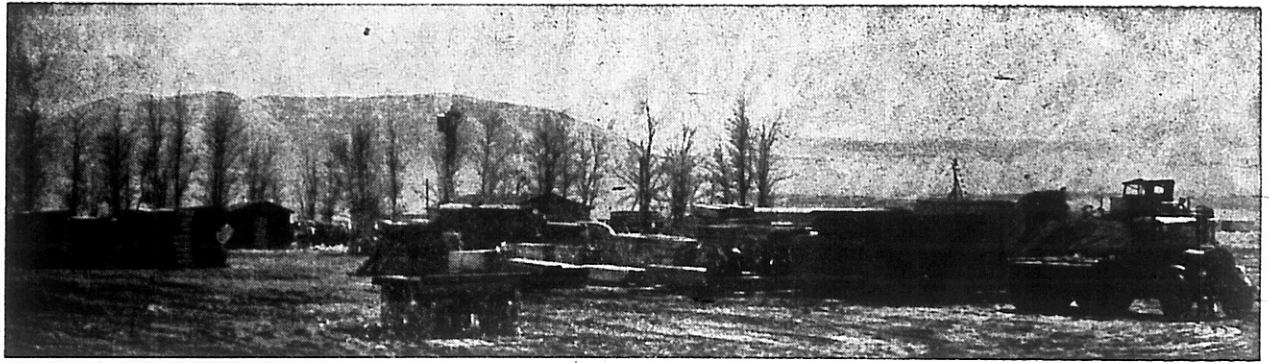
BOOM TOWN: Construction work begins on the new town for Japanese evacuees as trucks and tractors level off the ground and army of carpenters rushes building of barracks. Made simply in army style with rough boards covered with tar-paper an average of 39 barracks per day was built keeping more than 900 workmen busy. —Cut courtesy L. A. Times.
