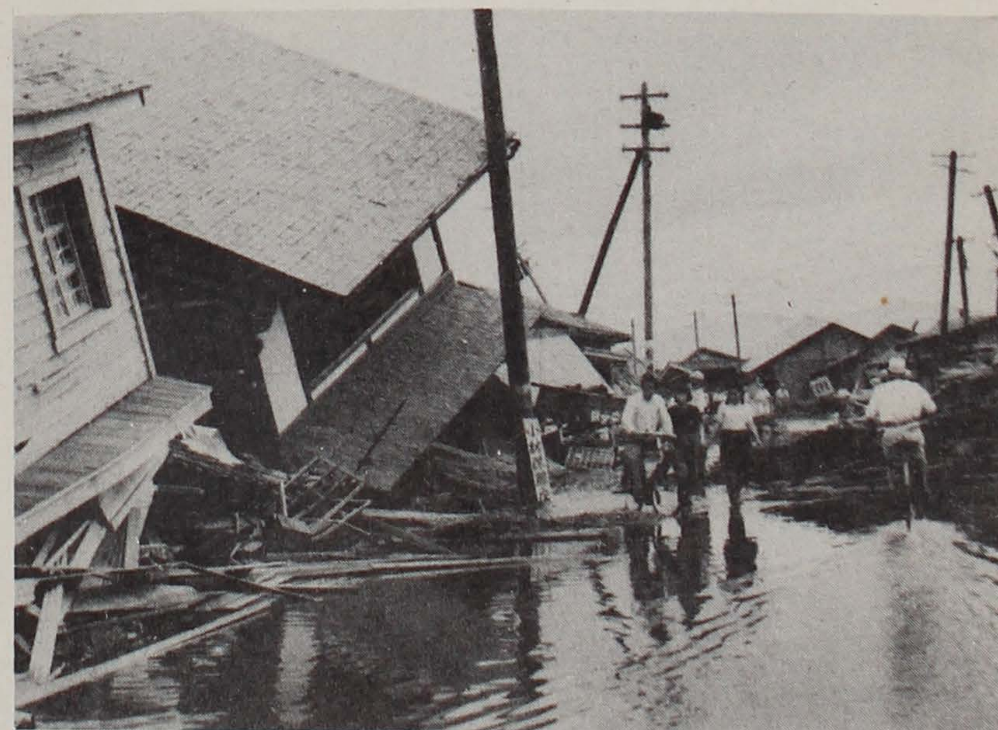
UNTOUCHED BY FIRE, these houses were nevertheless damaged by broken water mains which flooded flattened areas.
