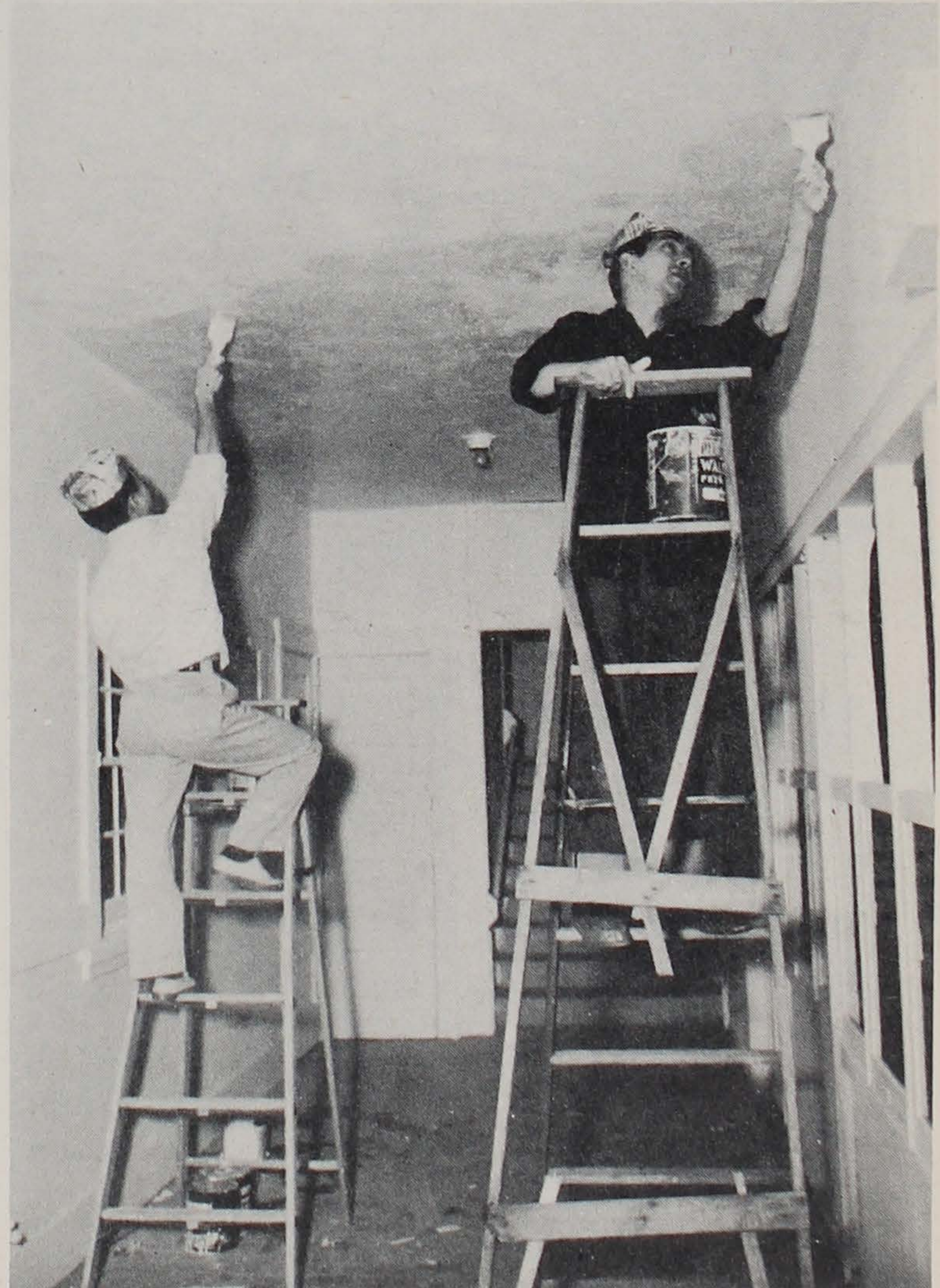
TWO MEMBERS of the Quixotics, George Akimoto (left) and Roy Uno, give neglected building much needed paint job.
