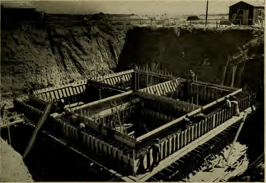
FIGURE 144: Deep below the sod of Heart Mountain Relocation Center, near Cody, Wyoming, once pounded by buffalo herds, rise the forms of reinforced concrete to house Imhoff or sanitary tank.
