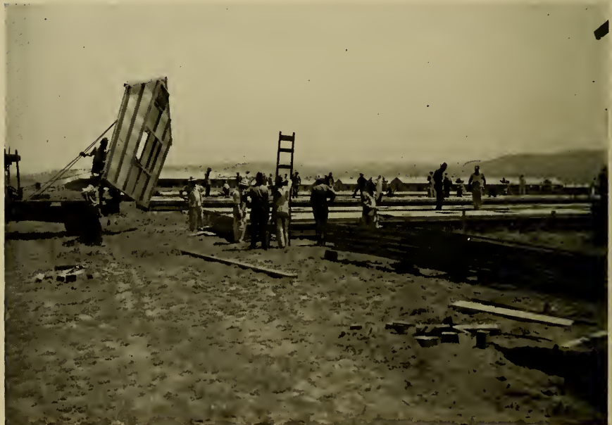
FIGURE 143: Buildings were put together in sections in a central construction area and these sections hauled by truck to the building site.
