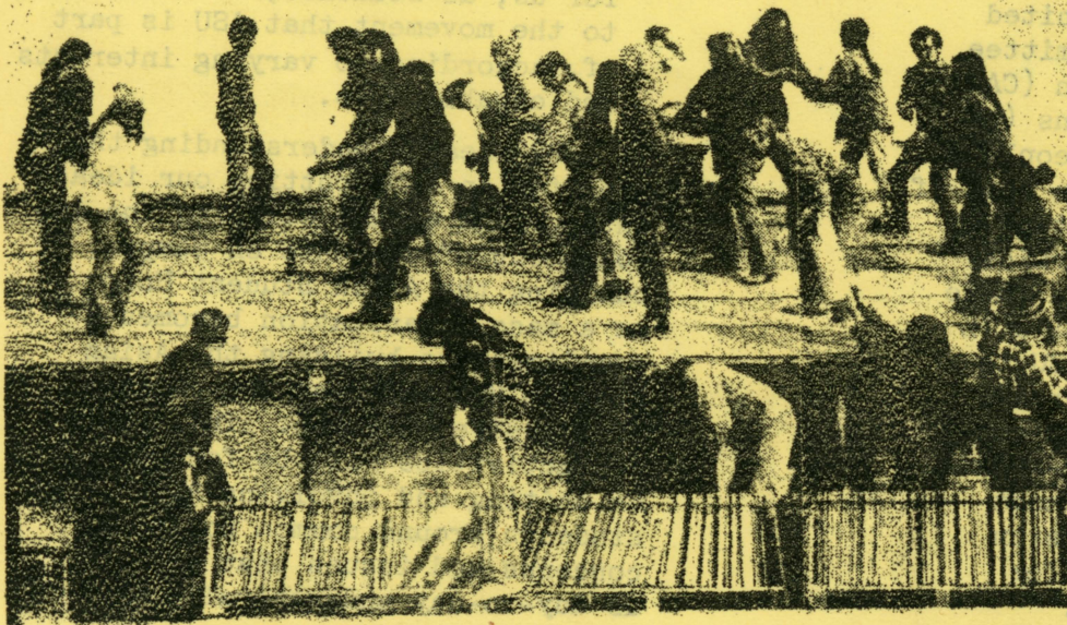
A work brigade at Agbayani Village - assisting in laying tiles on the roof.
