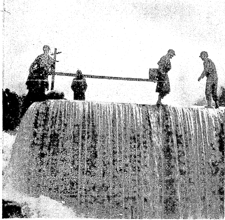
United States Army Engineers were called upon by the State Game Department yesterday to remove an obsolete power dam on the Tilton River at Morton, Lewis County. This photograph shows soldiers crossing the dam to place explosives.
