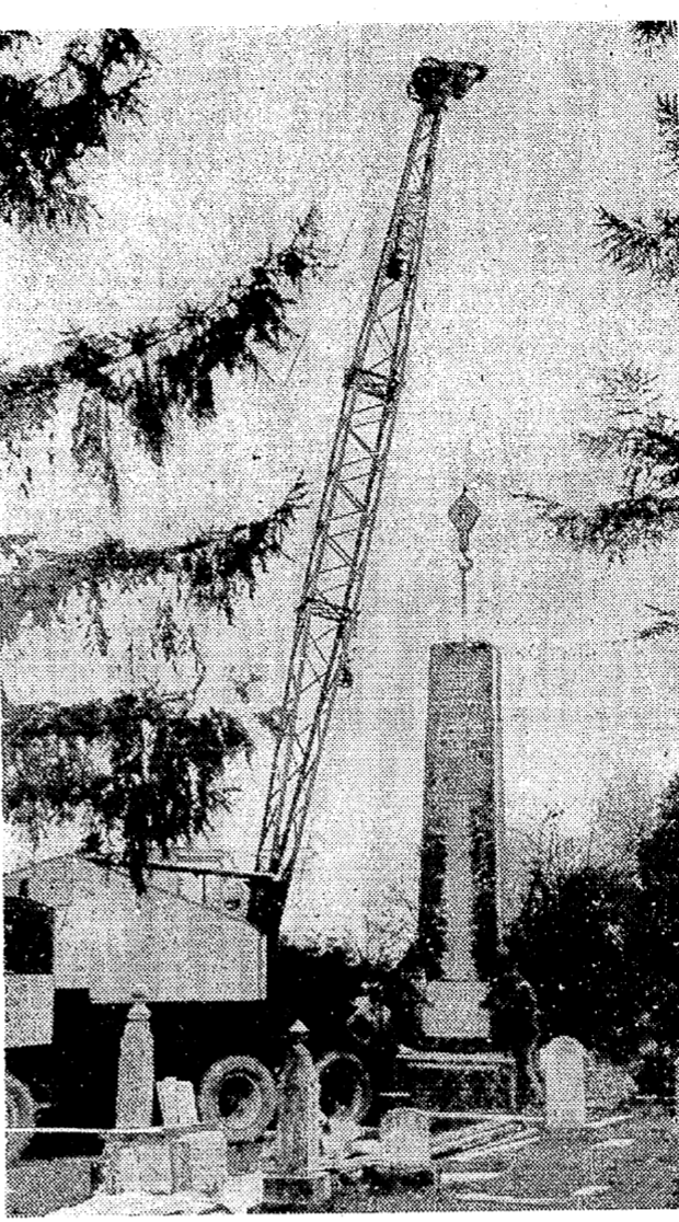
IN MEMORIAM: A crane lowered into position at Lake View Cemetery a granite memorial to 54 Seattle Nisei war dead.
