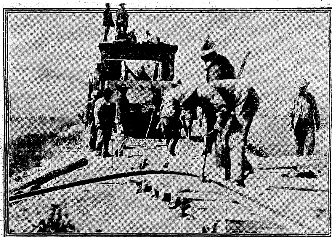
Copyright, 1914, by International News Service. REPAIRING RAILROAD AT TORREON. When the Federals retreated from their advanced positions into Torreon, they destroyed the railroad communication, so far as possible. In order to get his supply trains to the front, Villa was compelled to repair these lines. The photograph shows the rebel engineering corps repairing a section of train under the protection of a cannon mounted on the armored repair car.
